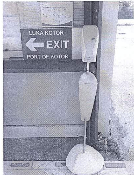
Figure 7 – Touchless Disinfectant Dispenser (Floor-disinfect) (Location: Port of Kotor administration)
